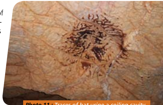
Photo 11 : Traces of bat urine on a ceiling cavity.
